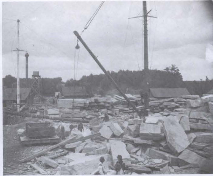
Moving and stacking slabs of Potsdam sandstone. (Courtesy of the St. Lawrence University Archives)
