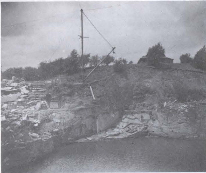
A worksite along the Racquette River. (Courtesy of the St. Lawrence University Archives)
